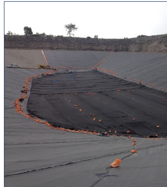
Above: Storage facility incorporates a high density polyethylene (HDPE) geomembrane liner underlain by a clay liner.
